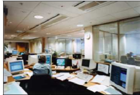
Example of a chilled beam installation. (Picture courtesy of Trox Brothers Limited.)
