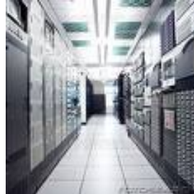
Tenant Computer server rooms
